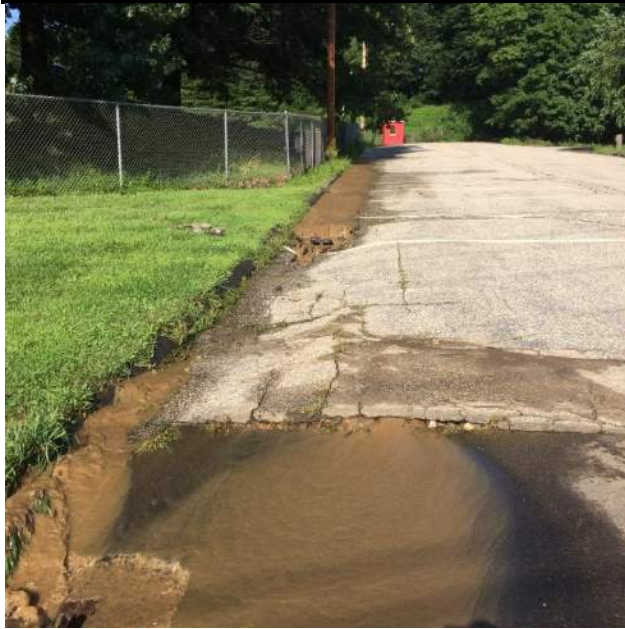
Run off at library parking areas
