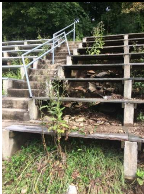
Wash out at home bleacher
