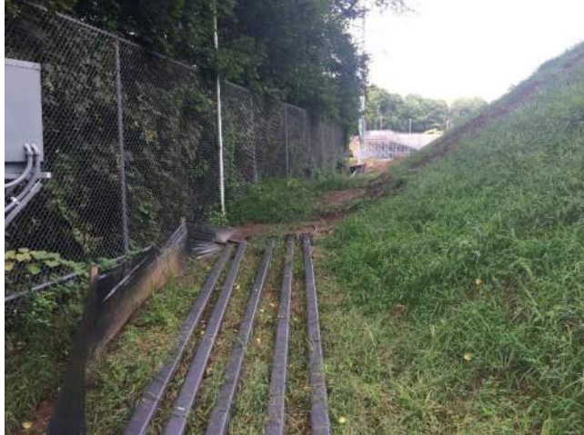
Slough at west of Stockpile (note buried silt fence)
